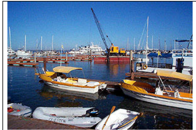
Looking out from the Marina office the construction on the new finger of B dock can be seen in front of the crane.
