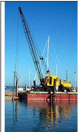
The crane on the floating platform used in construction. (click to enlarge)
